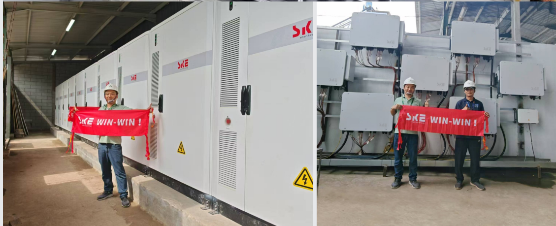
Indonesia Commercial&Industrial BESS 2.15MWh
